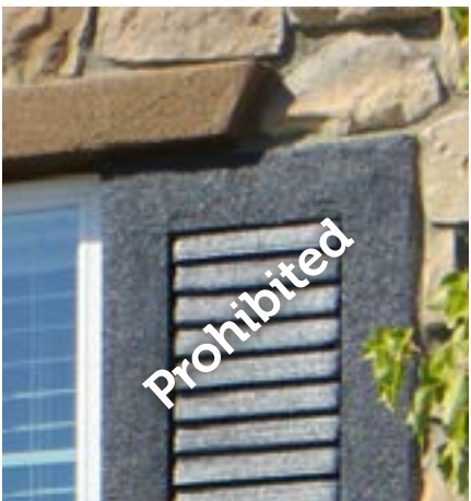
Example of prohibited embedded shutter
