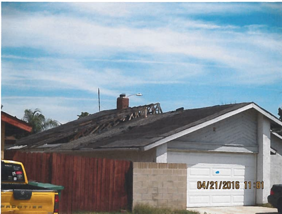
No roofing material, damaged/missing roof and no weather protection.
