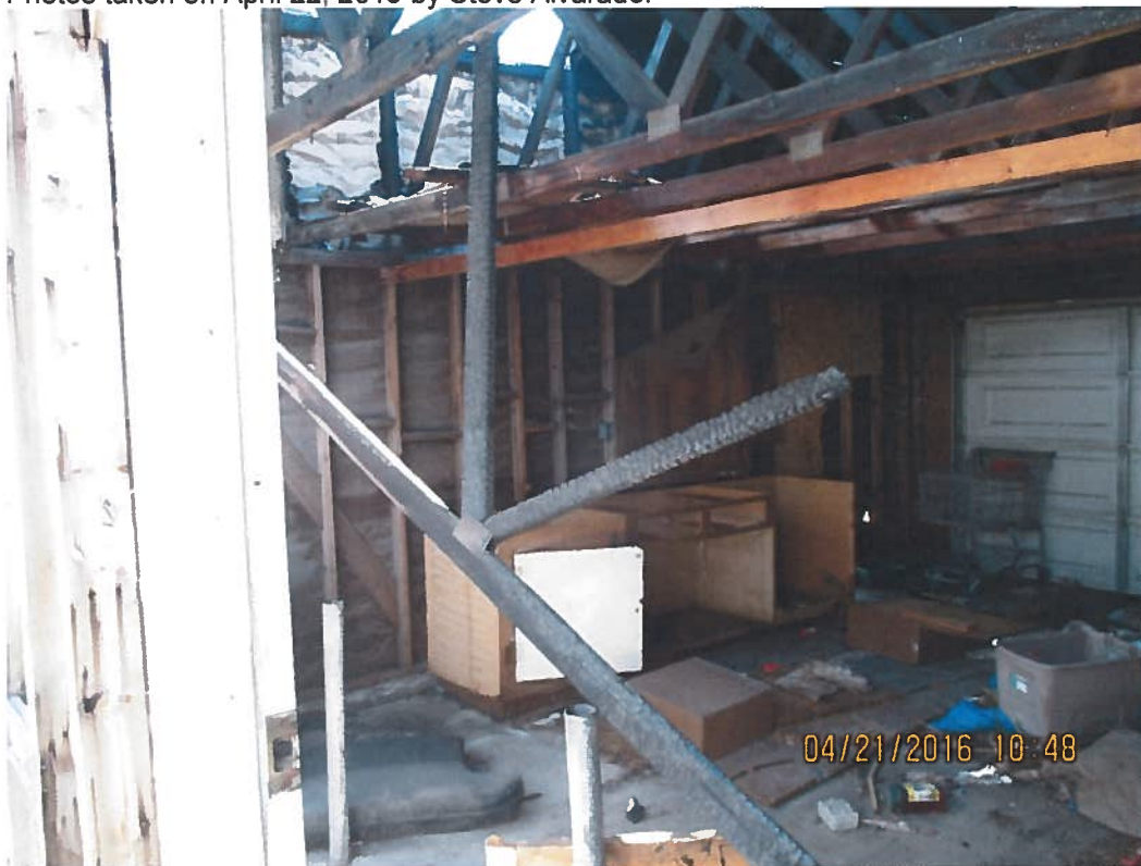
Massive charring on roof truss system
