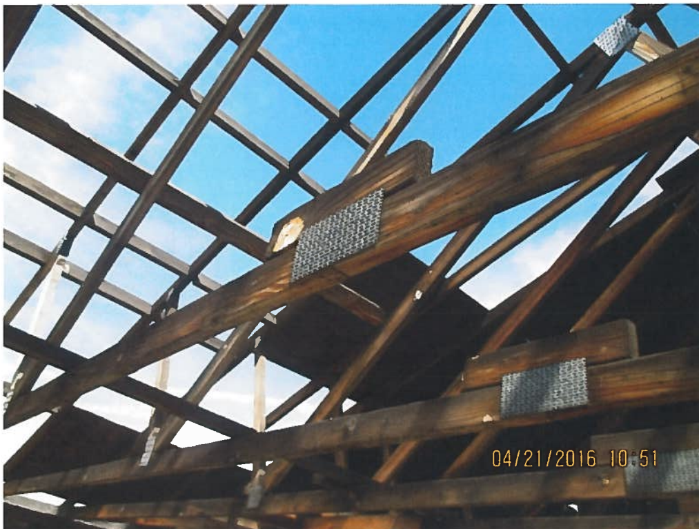
Non-engineered trusses with weathering and no weather protection.
