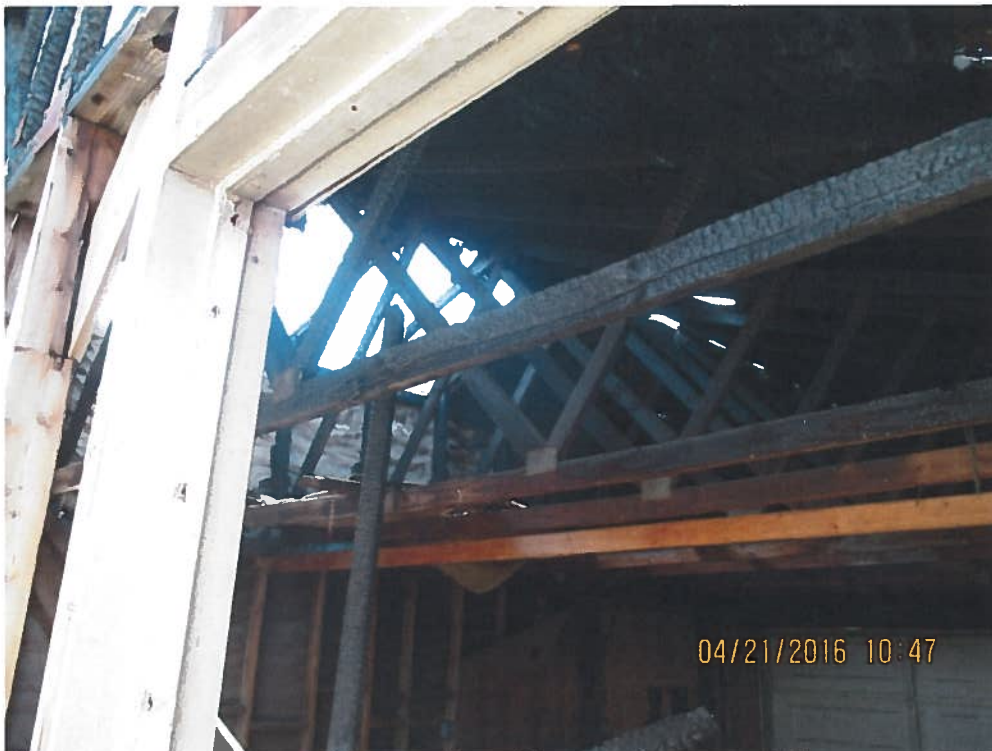
Burnt and charred roof truss and roof sheathing, no weather protection.
