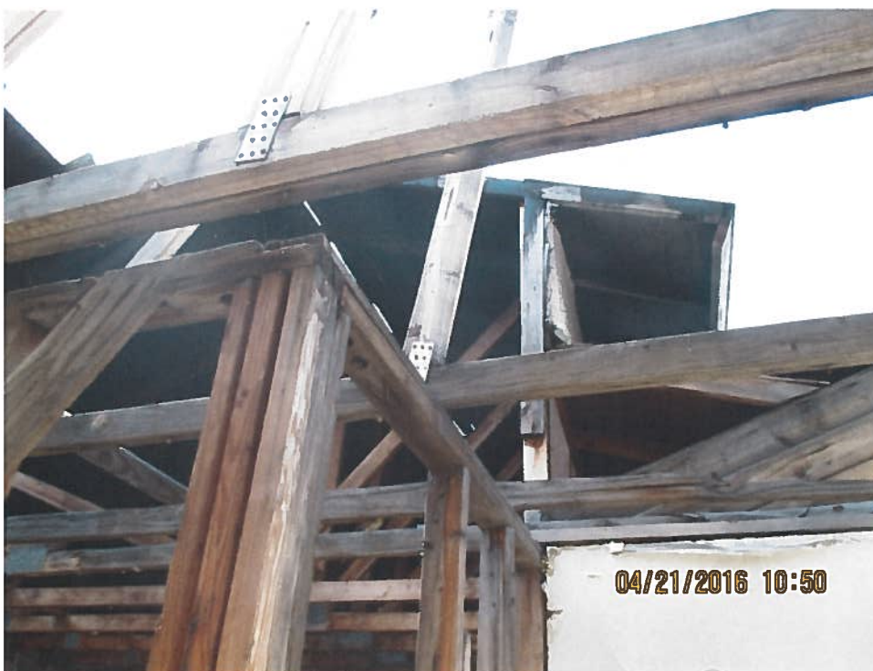
Weathered framing members.
