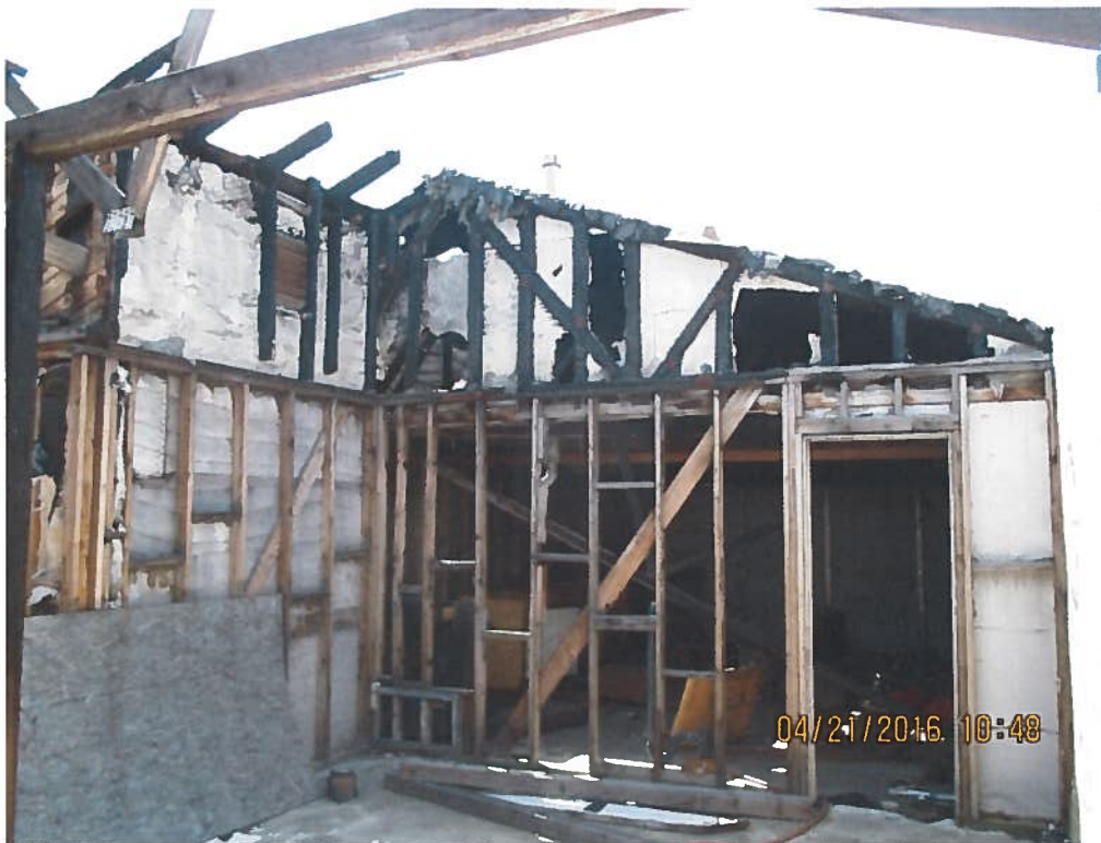
Fire damage and missing roofing system.
