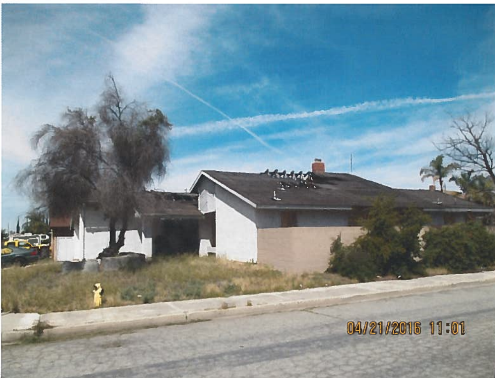
No roofing material, damaged/missing roof, no weather protection and overgrown vegetation.
