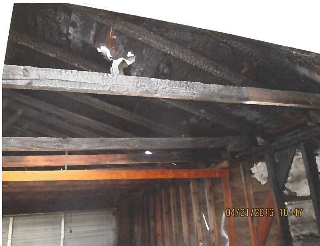
Burnt and charred roof truss and roof sheathing, no weather protection.
