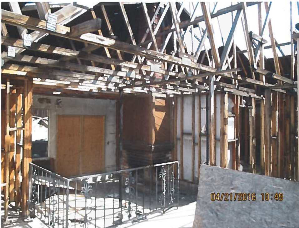
Non-engineered and unpermitted roof trusses.
