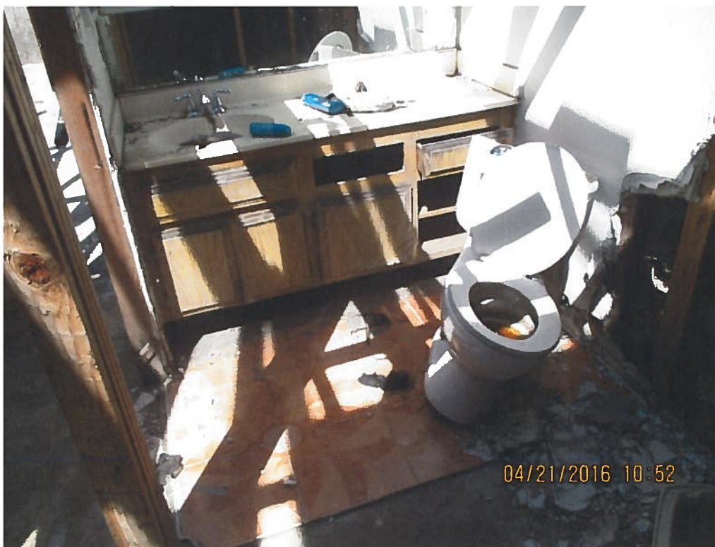
No plumbing fixtures with hot or cold running water.
