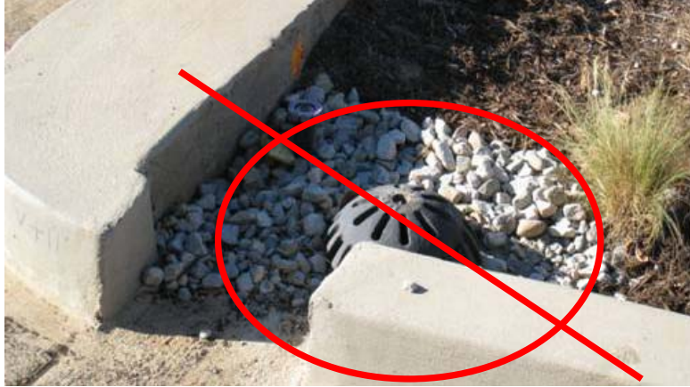
Figure 6: Incorrect Placement of an Overflow Inlet.
