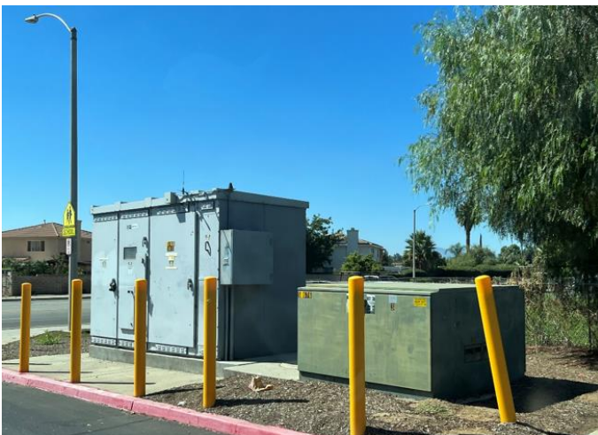
Electrical box on the corner – next to truck lane.
