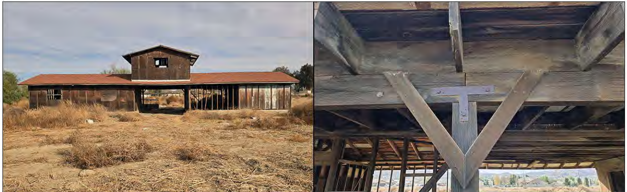
Barn. Left: southern façade, view to the north; right: structural framing, view to the north
